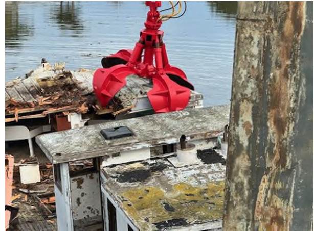
Figure 8. The Commission's contractor demolishing the Vaquero II in place before disposal. Photo credit: Lind Marine, LLC
