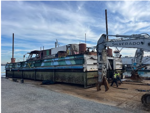
Figure 7. The Commission's contractor removing the floating barge from the water at its pier. Photo credit: Silverado Contractors, Inc.
