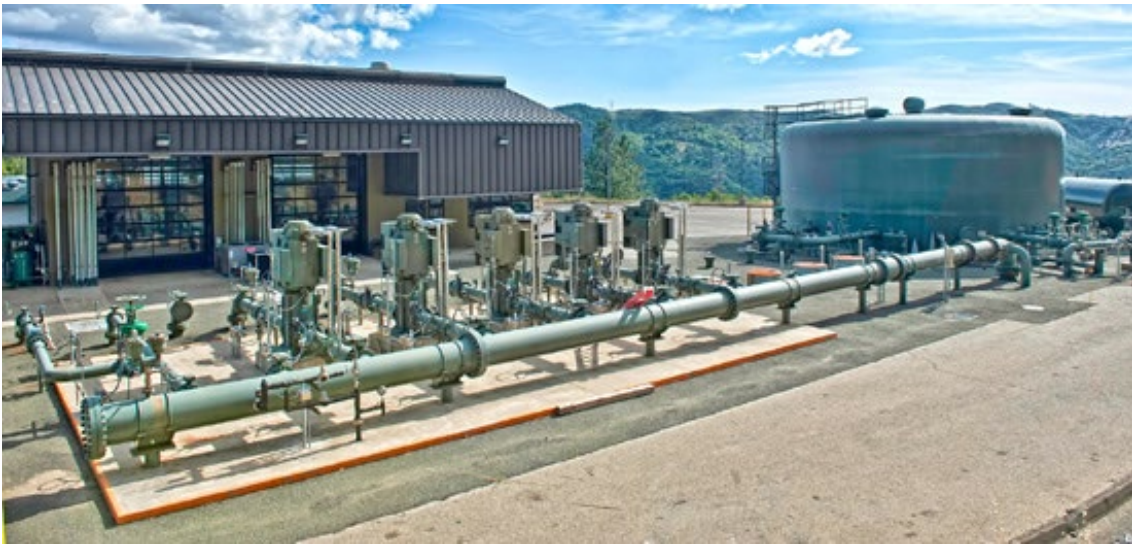
Figure 3: Santa Rosa Geysers Recharge Project, one of two large-scale recycled water injection projects at The Geysers, delivers and distributes approximately 11 million gallons of recycled water daily. Photo by John Grice, courtesy of the Calpine Corporation.
