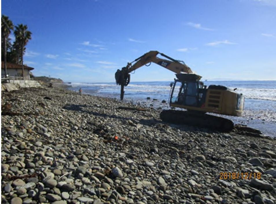
Figure 8. H Beam extracted near the Bacara Resort in Goleta, Santa Barbara County (photo by Commission staff).
