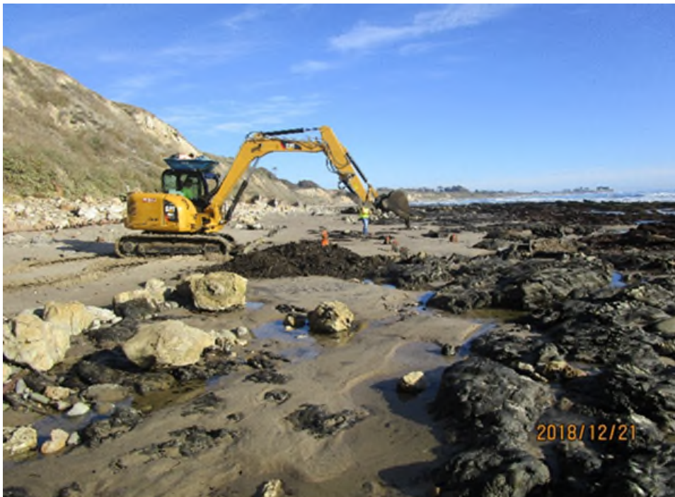
Figure 9. H Beam extracted near the Bacara Resort in Goleta, Santa Barbara County (photo by Commission staff).
