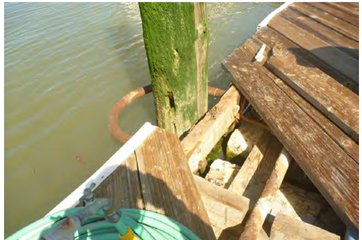
Dock B Mainwalk Framing Structure - Dry rot observed
