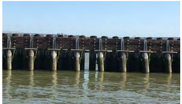
Breakwater Section B – Missing sheet pile
