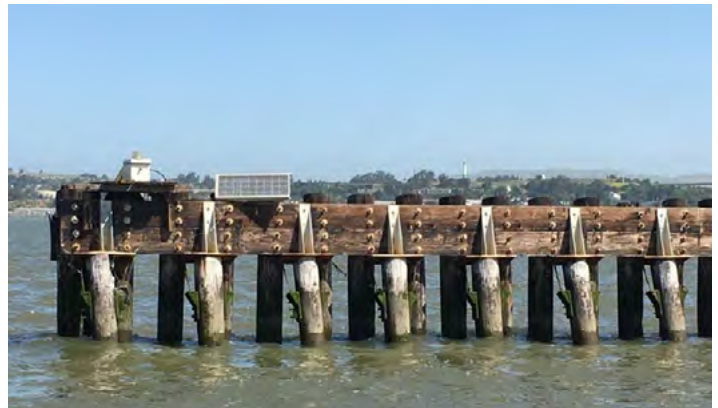
Breakwater Section C-1 – Missing sheet piles along full length
