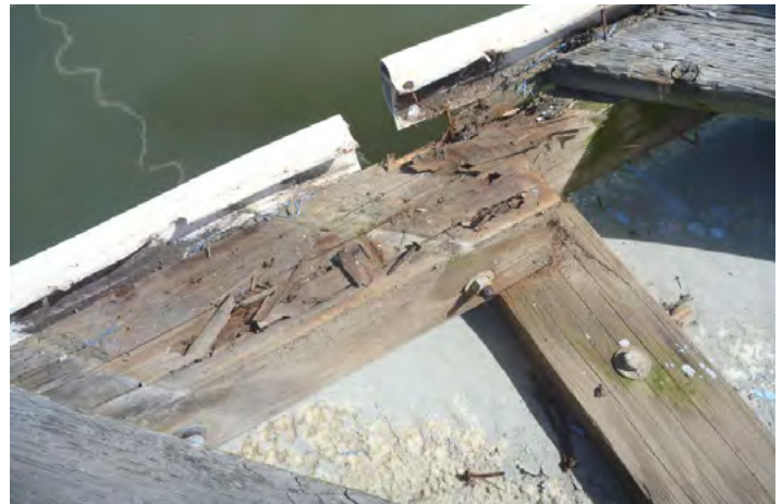
Dock D Finger Framing Structure - Broken deck boards and uneven walking surfaces
