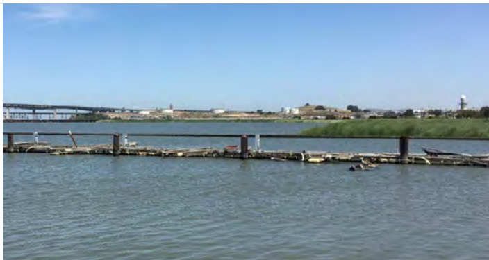
Breakwater Section D - Wall almost completely overtopped at +4-foot tide
