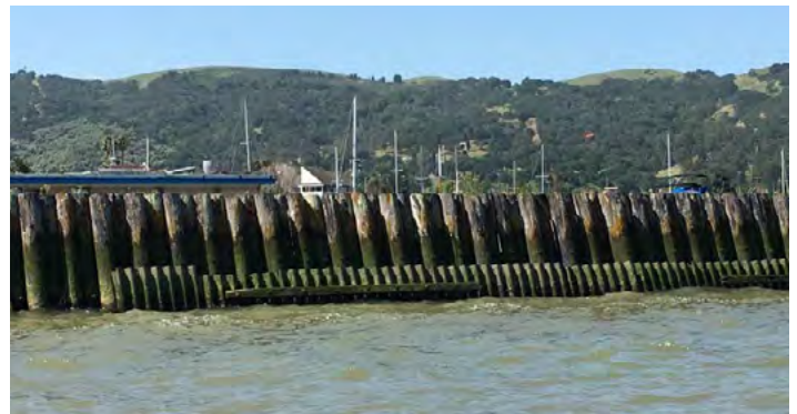
Breakwater Section C-2 – Missing/failing sheet piles, waler missing in several locations
