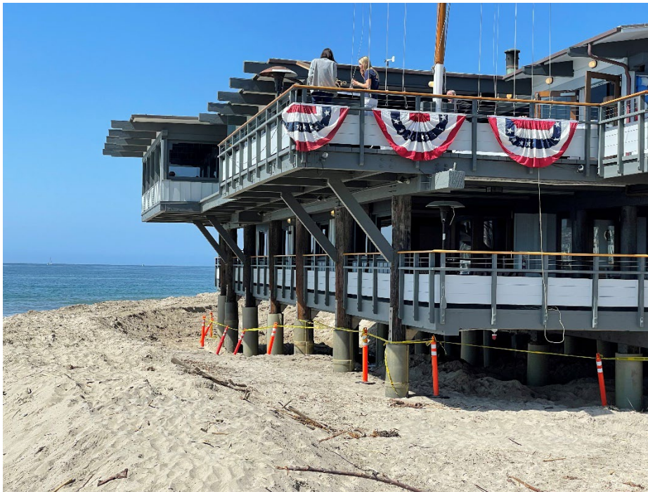
Figure 11: The Santa Barbara Yacht Club is elevated on pilings to accommodate some wave run-up and flooding. However, it still experienced structural damage from large waves in January 2023. Credit: Michael Wells
