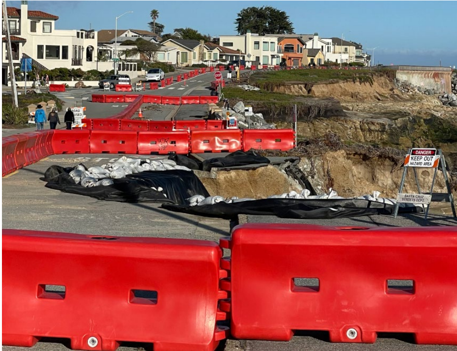
Figure 2: Major erosion from a large storm caused West Cliff Drive in Santa Cruz to close to traffic. Credit: Michael Wells
