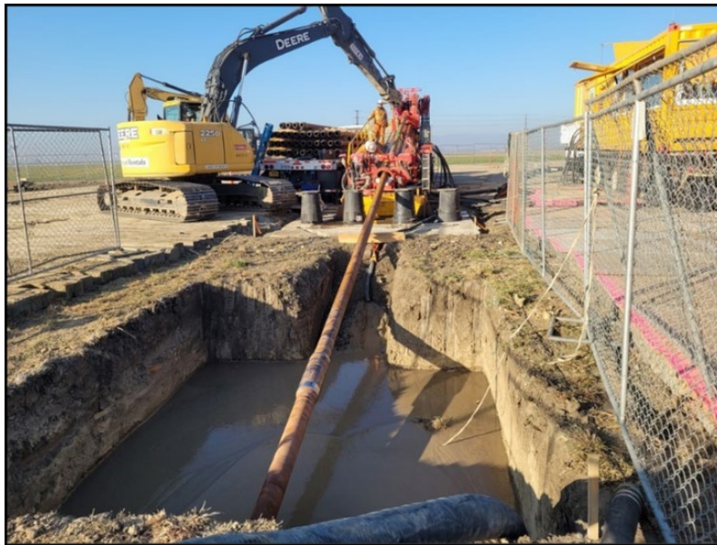
Figure 2-7. Photograph of an Example Drilling Rig and Entry Pit from a Previous Unrelated Project
