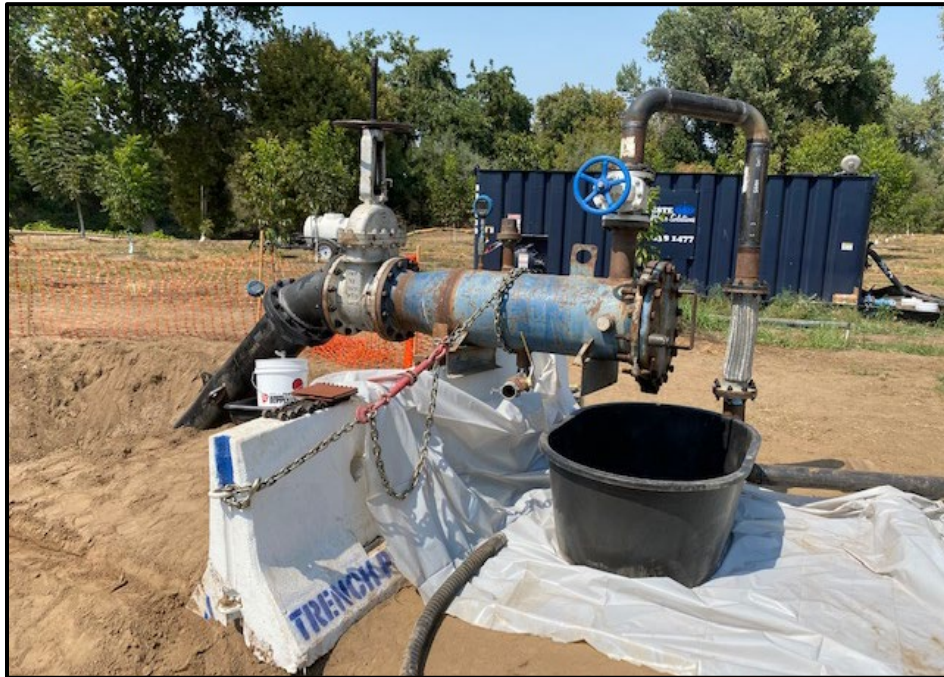
Figure 2-22. Photograph of a Typical Pig Receiver and Associated Equipment
