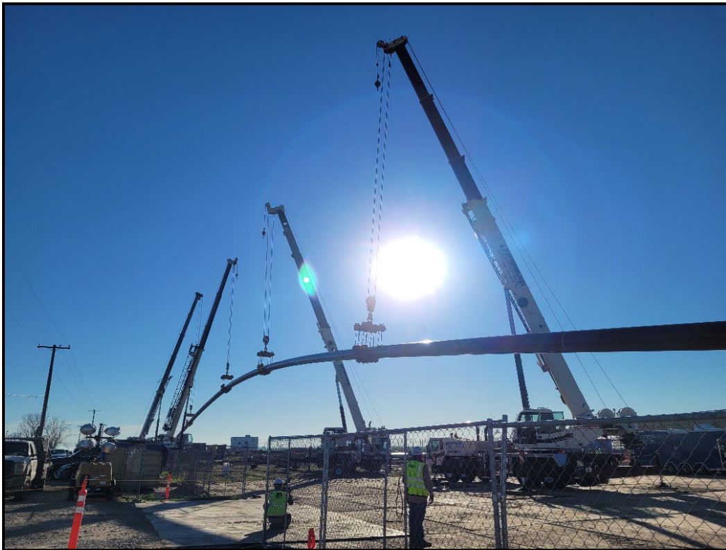
Figure 2-8. Photograph of an Example Cranes with Cradles Supported Pipeline (24-inch Diameter) During Pullback
