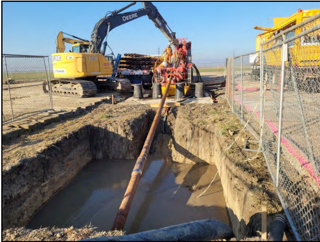
Figure 2-7. Photograph of an Example Drilling Rig and Bore Pit from a Previous Project
