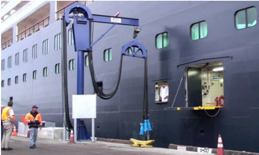
Figure 31 Use of new side port for plugging in passenger ship in San Diego (image, Port of San Diego)
