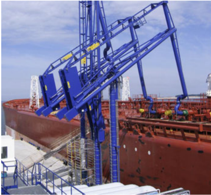
Figure 27 Loading arms to tanker
