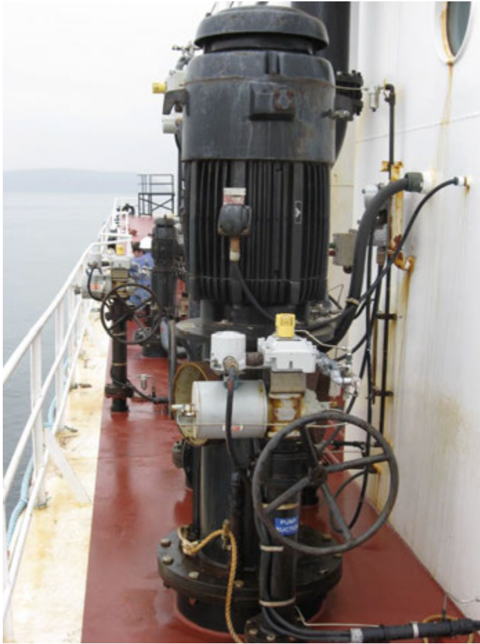
Figure 17 Deepwell pump as installed, with discharge flange on Main Deck
