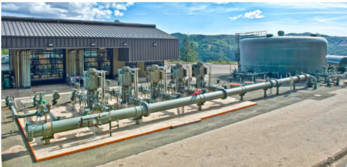
Figure 3: Santa Rosa Geysers Recharge Project, one of two large-scale recycled water injection projects at The Geysers, delivers and distributes approximately 11 million gallons of recycled water daily. Photo by John Grice, courtesy of Calpine
