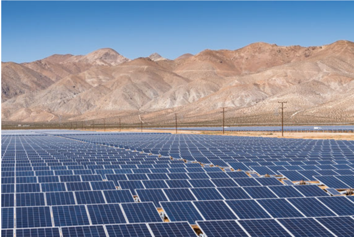
Figure 10. Beacon Point Solar Panel Array in Barstow, California. Photo courtesy Los Angeles Department of Water and Power/photographer Chris Corsmeier.
